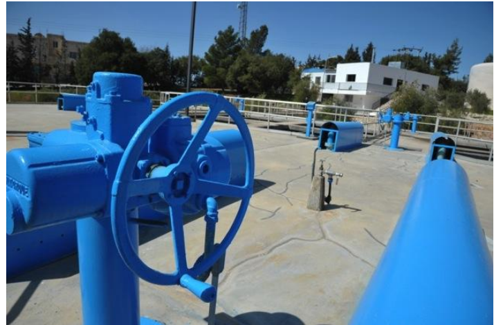
Many plants use state-of-the-art technology, such as these electro-mechanical installations at Miyahuna/Zai Water Treatment Plant. Operator certification training helps engineers and technicians to remain up-to-date in this dynamic industry.
